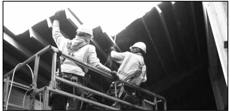
Workers are doubling the dry fertilizer storage at our Randolph agronomy plant.
